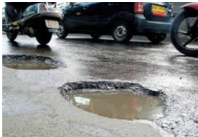
Fig 1. Condition of Indian roads with potholes.
