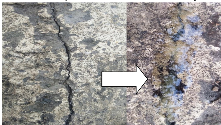
Cracked floor surface
