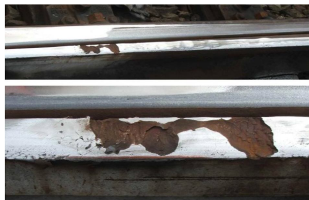
Fig 2:squats on railway track
