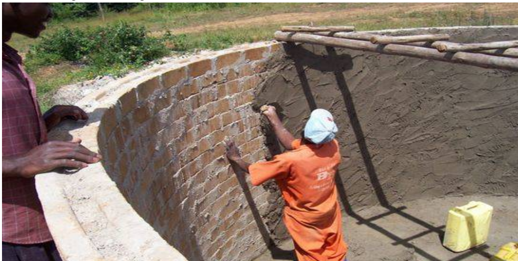
Fig. 1.1 Circular Water Tank
