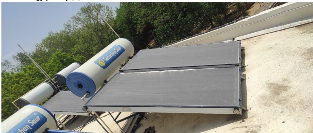
Fig.1: Setup of experimental solar water heater.
