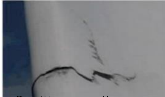
Figure 4(a): transverse cracking.
