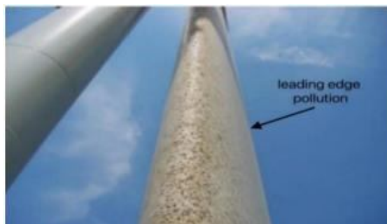
Figure 6(a): Pollution on wind turbine.
