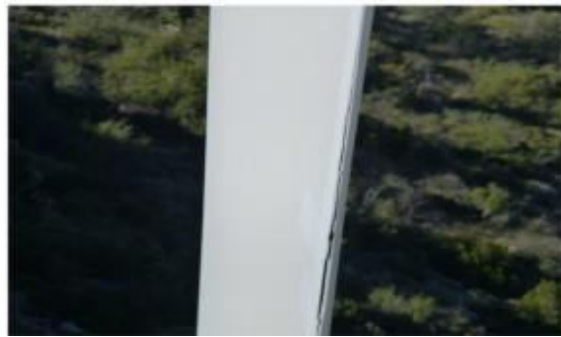
Figure 4(b): Longitudinal cracking.
