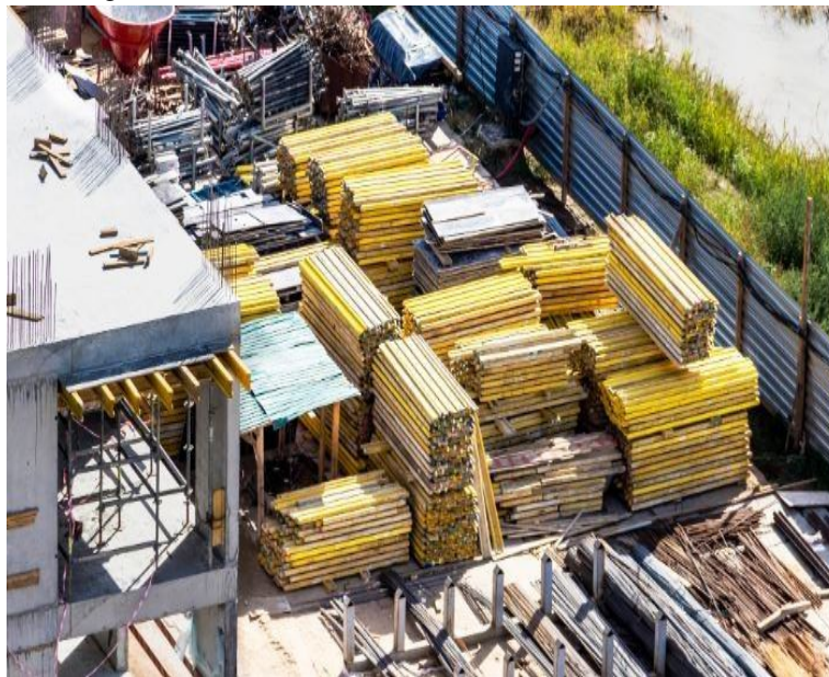
Fig 3. Storage of Construction Materials
