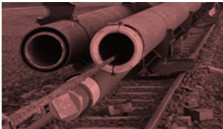
Fig. 1 Shows the utility of pipelines by the oil company
