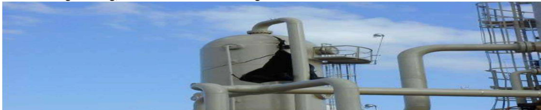
Fig. 2. Failure of pressure vessel during hydro Test.
