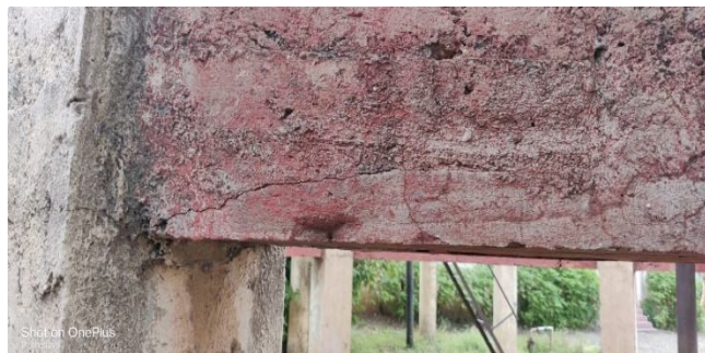
Figure 6 : Cracks in bracing
