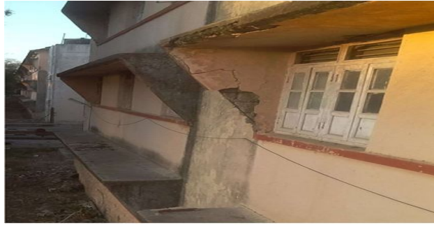
Figure 7: Cracks in chajja
