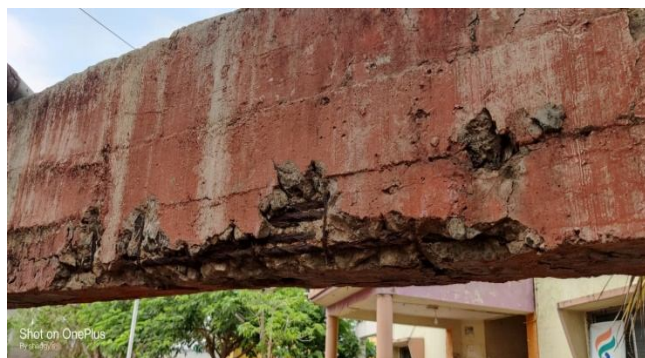
Figure 5 : Exposed and reinforcement at bottom of bracing
