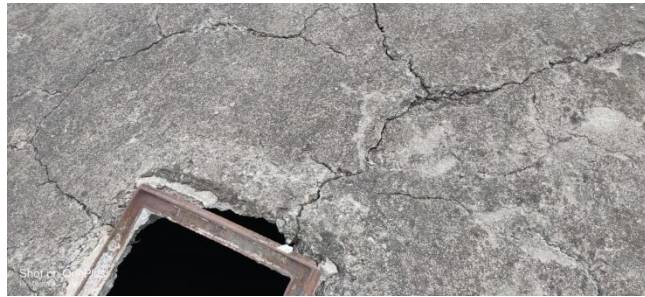
Figure 4: Cracks in slab of ESR
