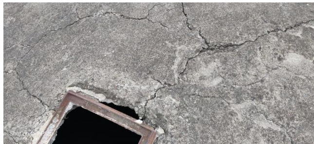
Figure 4: Cracks in slab of ESR
