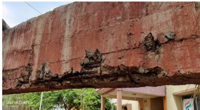
Figure 5 : Exposed and reinforcement at bottom of bracing
