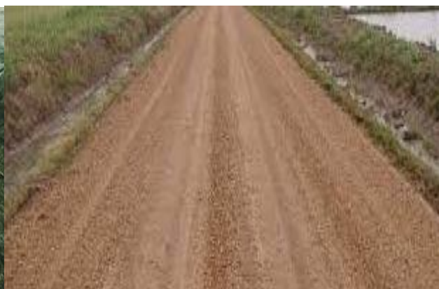
Figure 9 Formation of ruts in reinforced section
