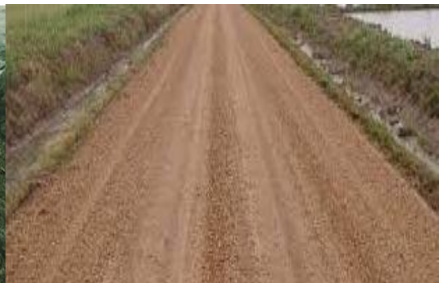
Figure 9 Formation of ruts in reinforced section
