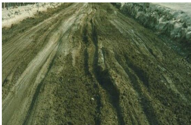
Figure 8 Formation of ruts in un reinforced section
