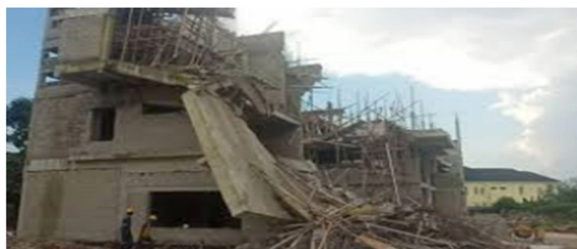
Figure 1.2: Two -Storey Building that collapsed in Abuja, Nigeria (2023)
