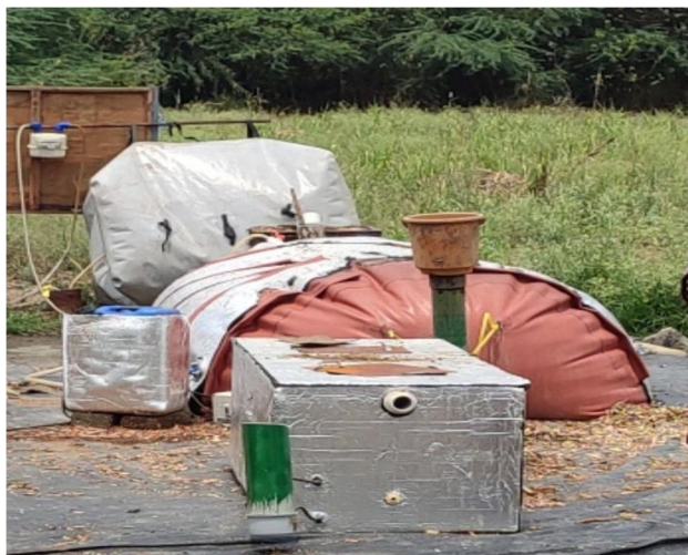
Image 2: Fixed Dome Plug Flow Digester (without Partition)
