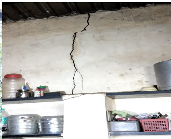
Fig. Vertical crack formation
