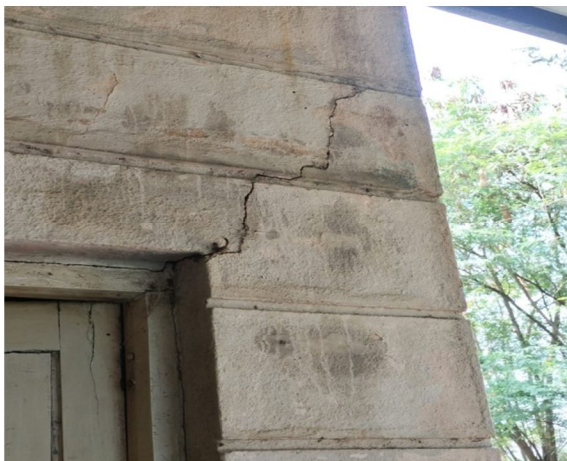
Fig. Diagonal crack formation
