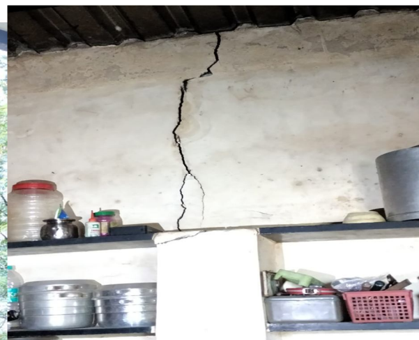
Fig. Vertical crack formation
