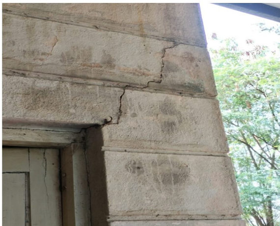
Fig. Diagonal crack formation
