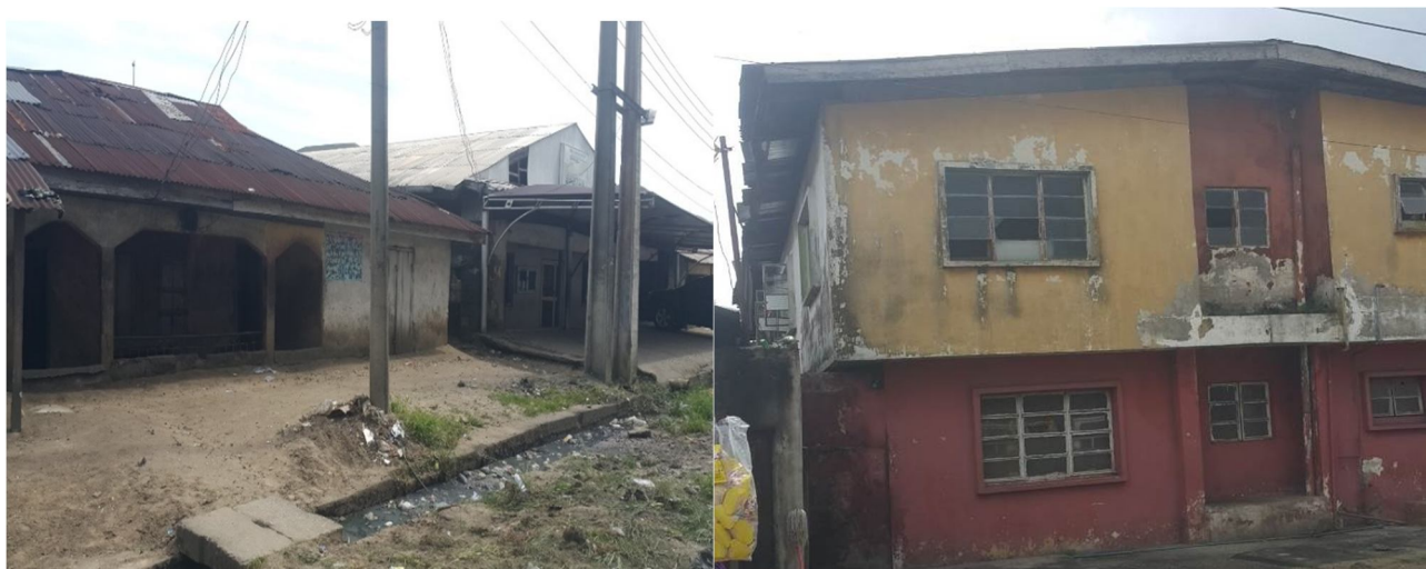
Figure 3: A building in the study area with dampened wall and poor design- floor level is lower than ground level. Figure 4: A building with faded wall paint and broken window glass.
