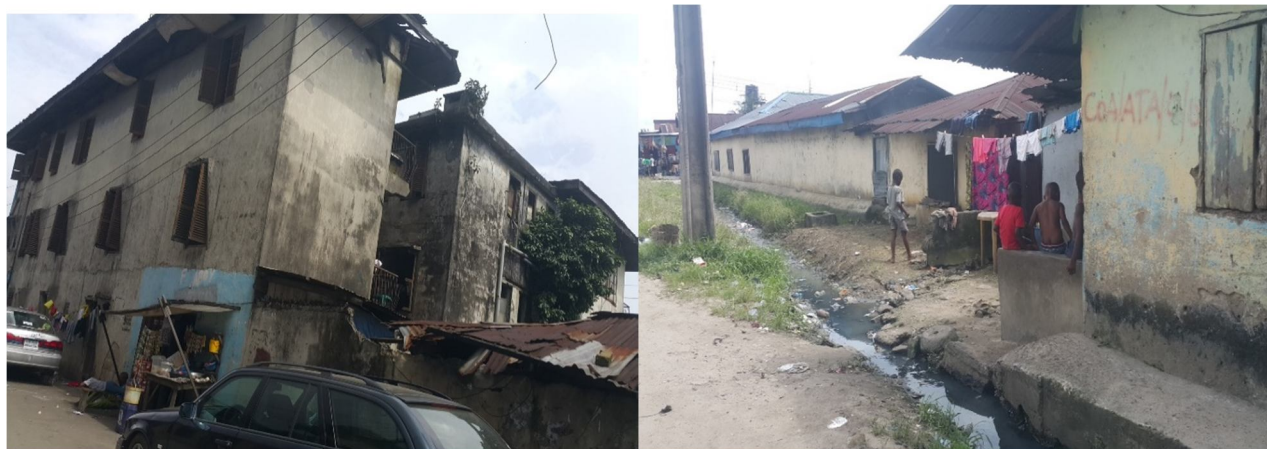
Figure 1: Water dampness caused by poor drainage facilities. Figure 2: A building in the study area with dampened wall
