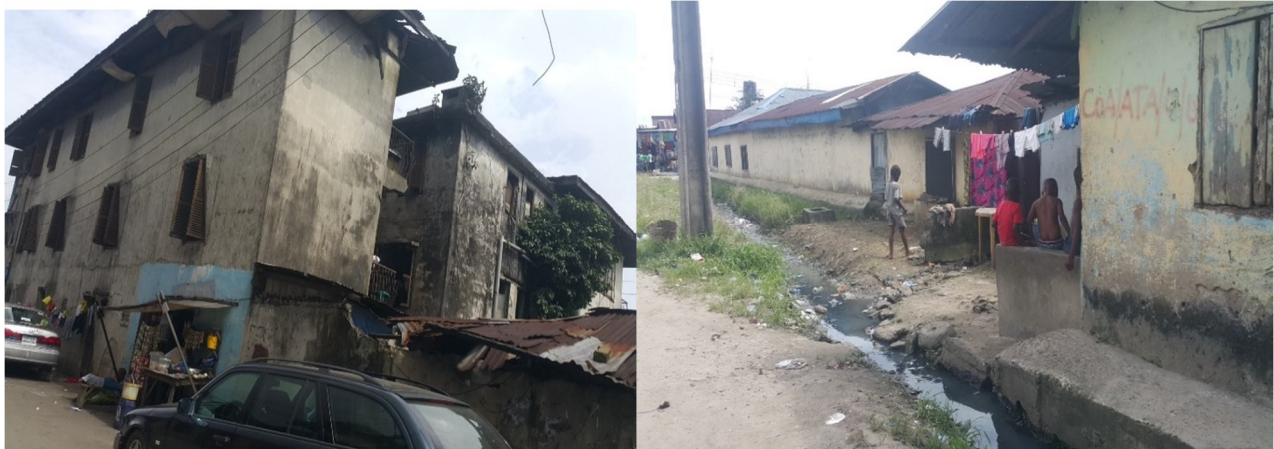
Figure 1: Water dampness caused by poor drainage facilities. Figure 2: A building in the study area with dampened wall
