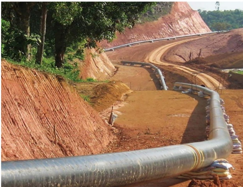
Fig. 2 – Bends in slurry pipelines.
