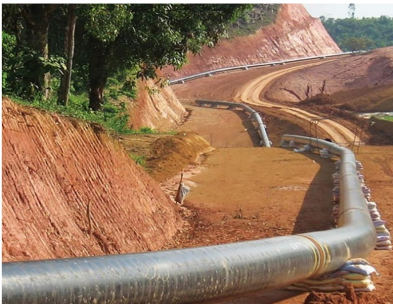
Fig. 2 – Bends in slurry pipelines.
