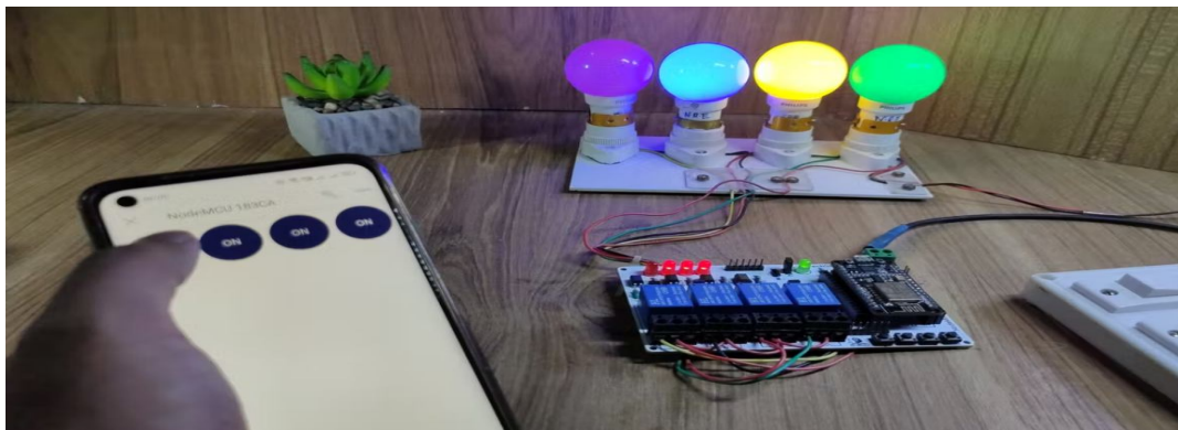
Fig. 7 Image of Remote Controlling of Lights Using a Mobile Application
