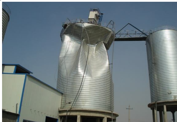
Fig. 1 Stages of Cement Silo Failure on Steel Structure
