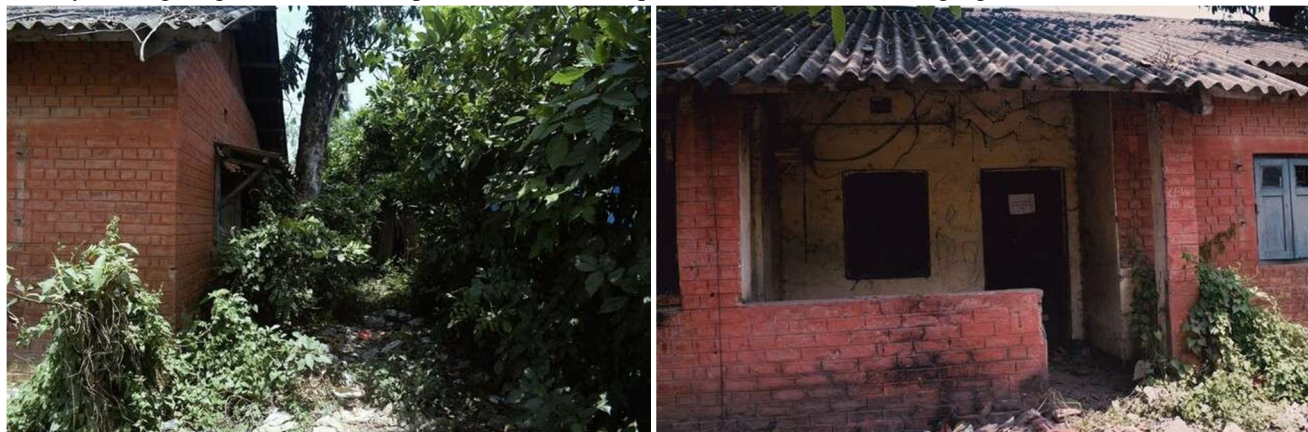
Fig. 10 Visuals showing dilapidated condition of the quarters around the neighbourhood
