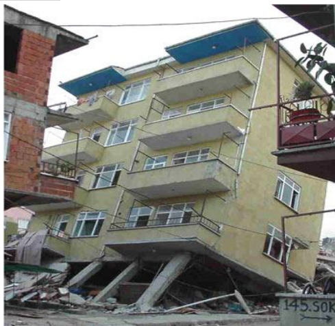
Soft Storey Failure of Building
