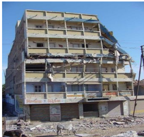
Soft Storey Failure of Building
