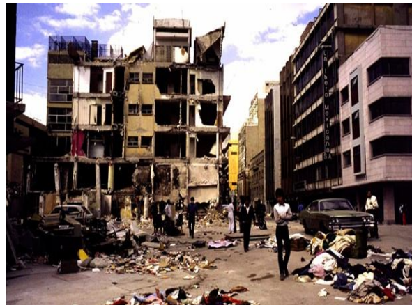
Collapsed buildings with mass irregularity
