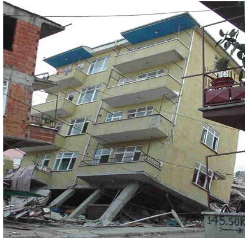
Soft Storey Failure of Building
