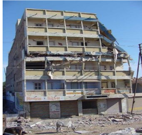
Soft Storey Failure of Building
