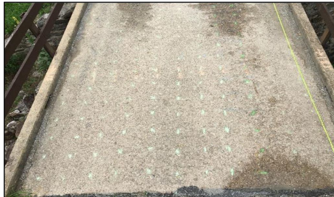
Figure 2. Visual evidence of loss of concrete surface.
