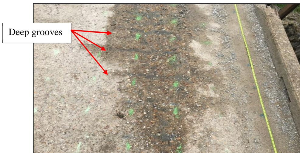
Figure 3. Visual evidence shows deep grooves. (Grooves about 3 inches deep cover over half of the bridge deck area)
