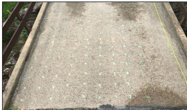
Figure 2. Visual evidence of loss of concrete surface.
