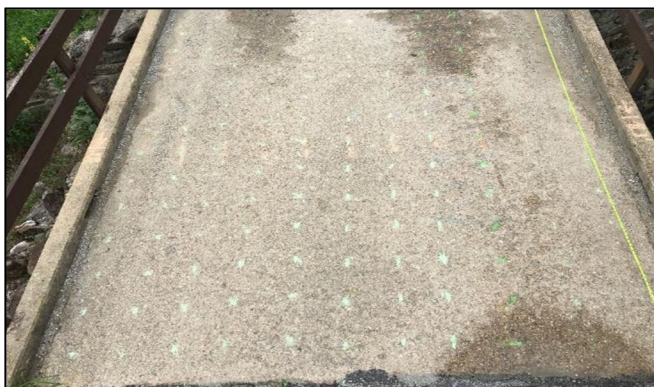
Figure 2. Visual evidence of loss of concrete surface.
