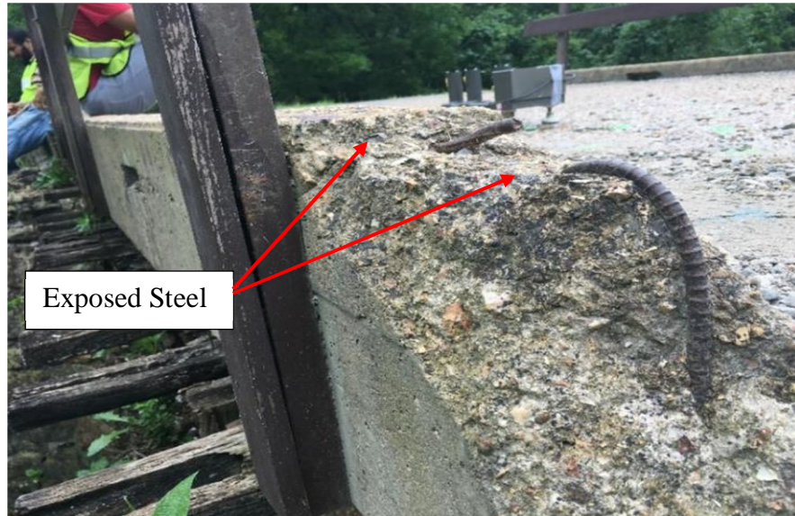
Figure 4. Visual evidence shows the exposed reinforcement steel bar. (In the picture is a corroded steel bars on the girder.)
