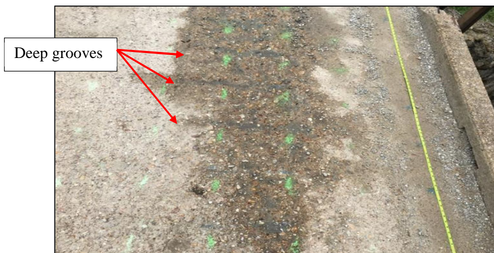
Figure 3. Visual evidence shows deep grooves. (Grooves about 3 inches deep cover over half of the bridge deck area)
