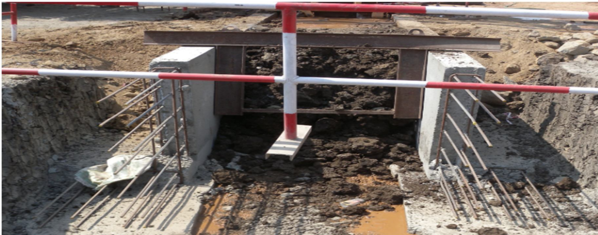
Fig 8. A view of Guide wall
