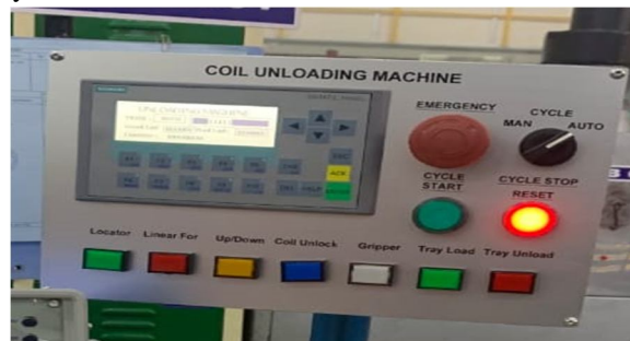
Fig 1.9 Output of coil unloading machine.
