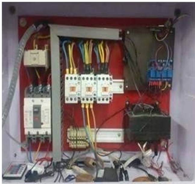
Figure 7(a). Inside the panel
