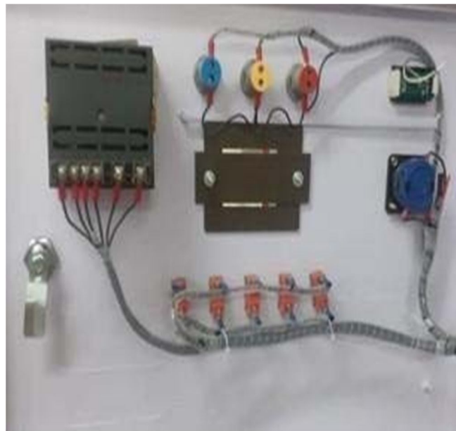
Figure 7(b) - Inside the panel
