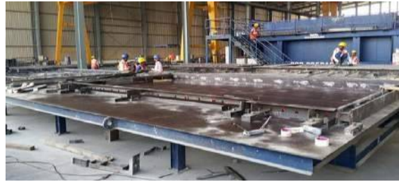
Figure 23: Tilting tables for horizontal production of precast wall panels
