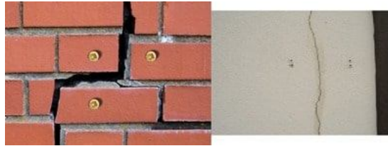
Fig.7: Installing three screws at right angle triangle to measure both shear and normal movement
