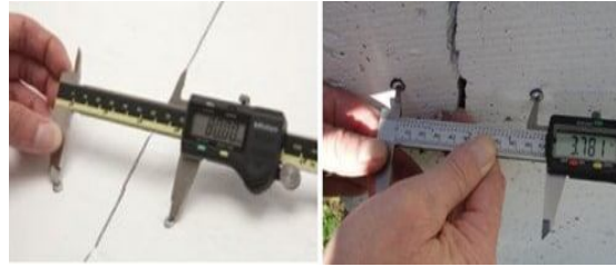
Fig.6: Measuring crack width using caliper by fixing its ends on the installed screws on each side of the crack
