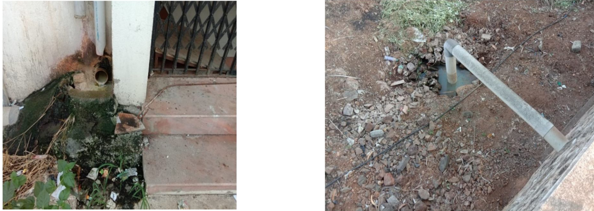
Fig.4.1 Waste water directly discharged into open land.
