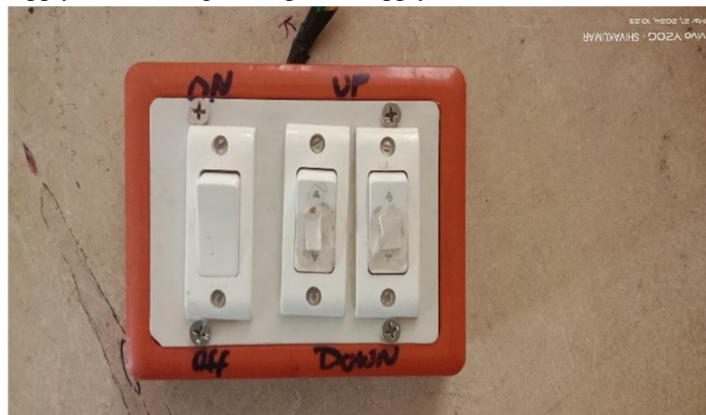
Fig:10. Switch Board
