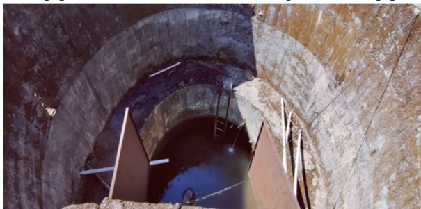
FIG 3. Existing Jack well
