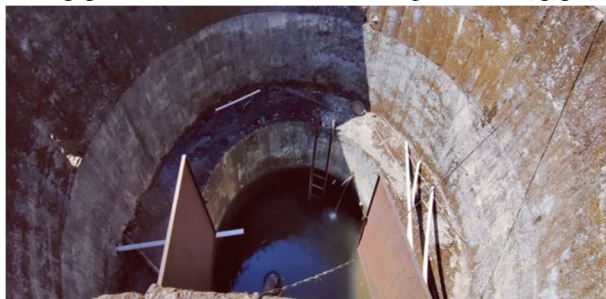
FIG 3. Existing Jack well
