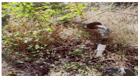
FIG 5. Existing Bore well
