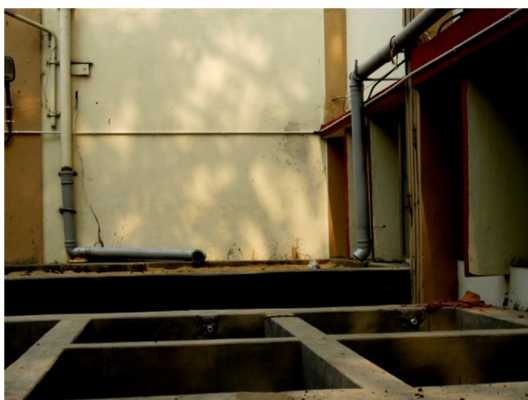
Rain Water Harvest System & Fish Tank
