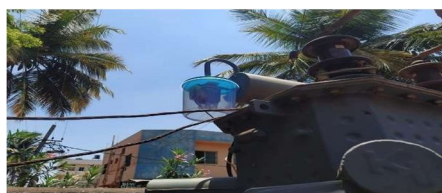
Fig.8 Project Model Tested and installed on 11KVTransformer in Campus
