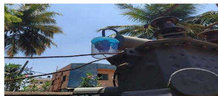
Fig.8 Project Model Tested and installed on 11KVTransformer in Campus
