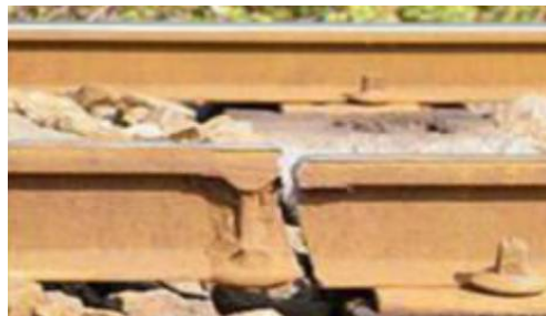
Figure 1. Railway Track Crack
