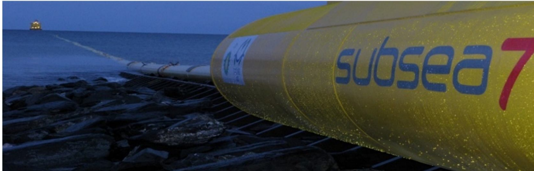
Fig. 1 Showing subsea export pipelines [6]
