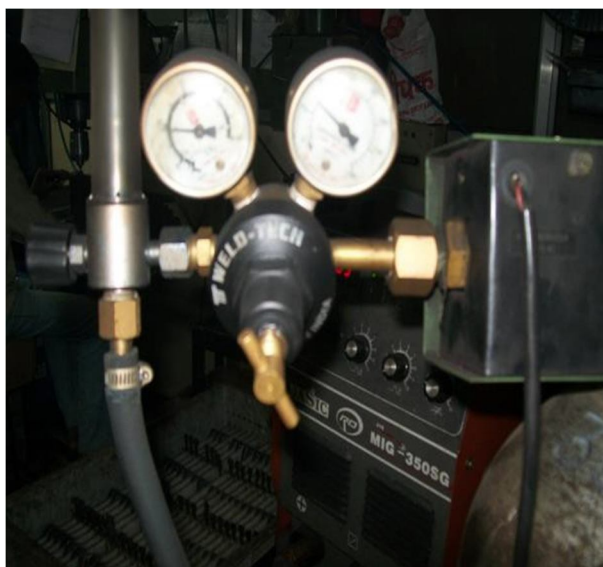
Figure 3: Gas Preheater and Pressure Regulator
