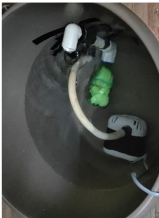
Fig 1.3 :- Filtered Water (After Filtration)
