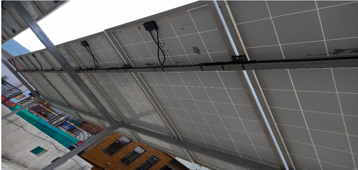
Figure 1: Solar Roof Power Generation
