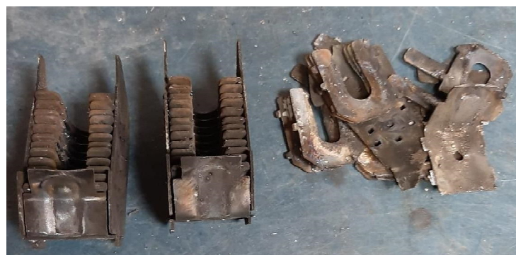
Fig. 5. Damage in Separators of Non-Limiter Circuit Breakers
