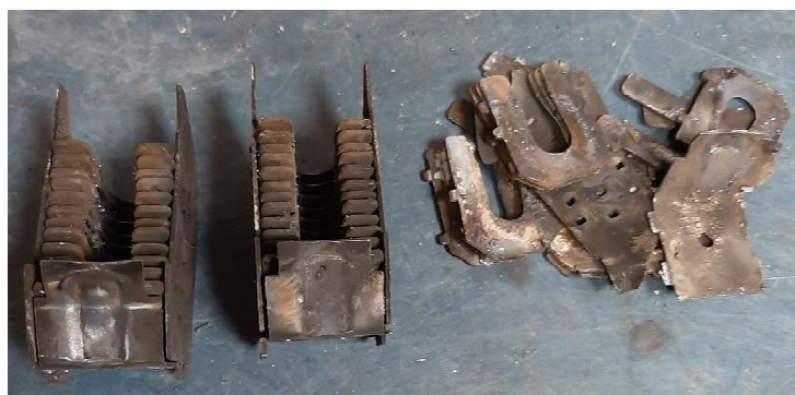
Fig. 5. Damage in Separators of Non-Limiter Circuit Breakers
