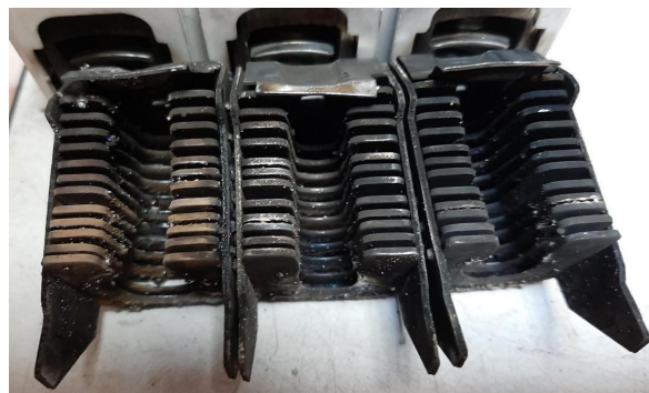
Fig. 7. Damage in Separators of Limiter-Equipped Circuit Breakers
