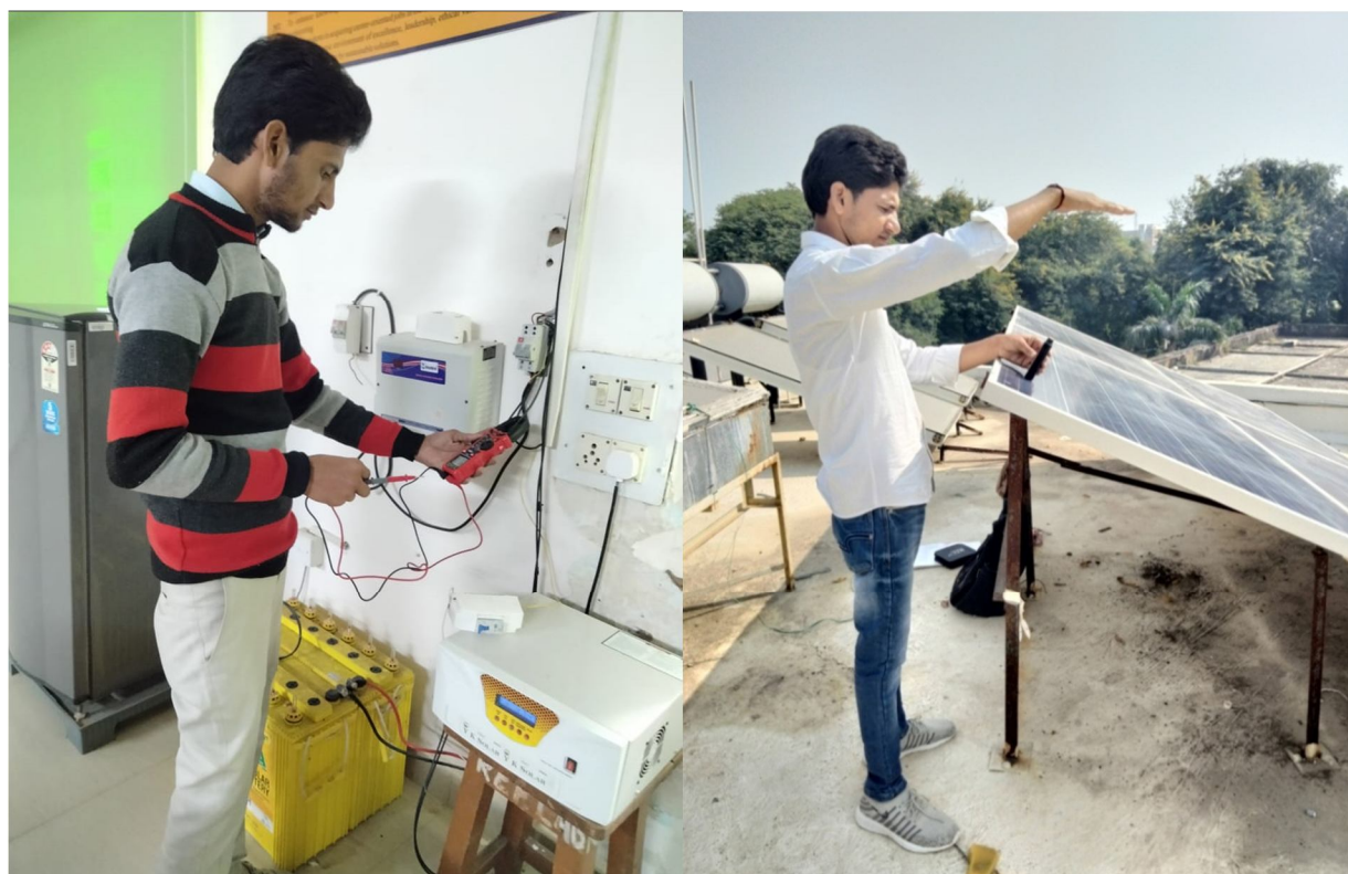
Fig.2 Photograph of PV panel and Battery – Inverter Arrangements
