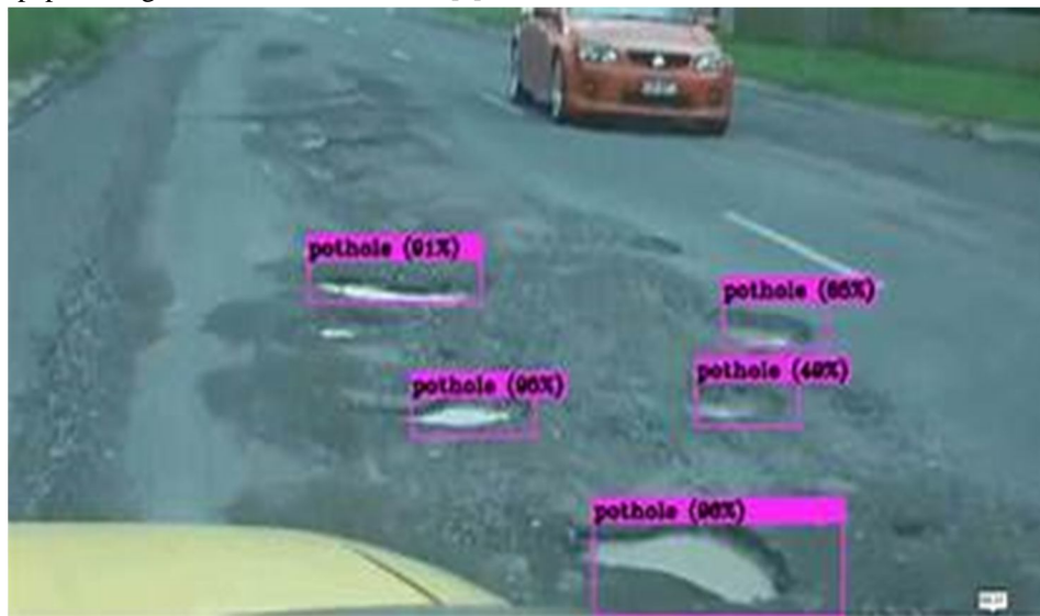
Fig : Pothole Detection
