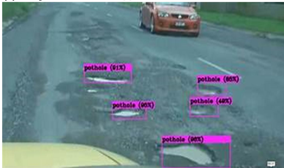
Fig : Pothole Detection
