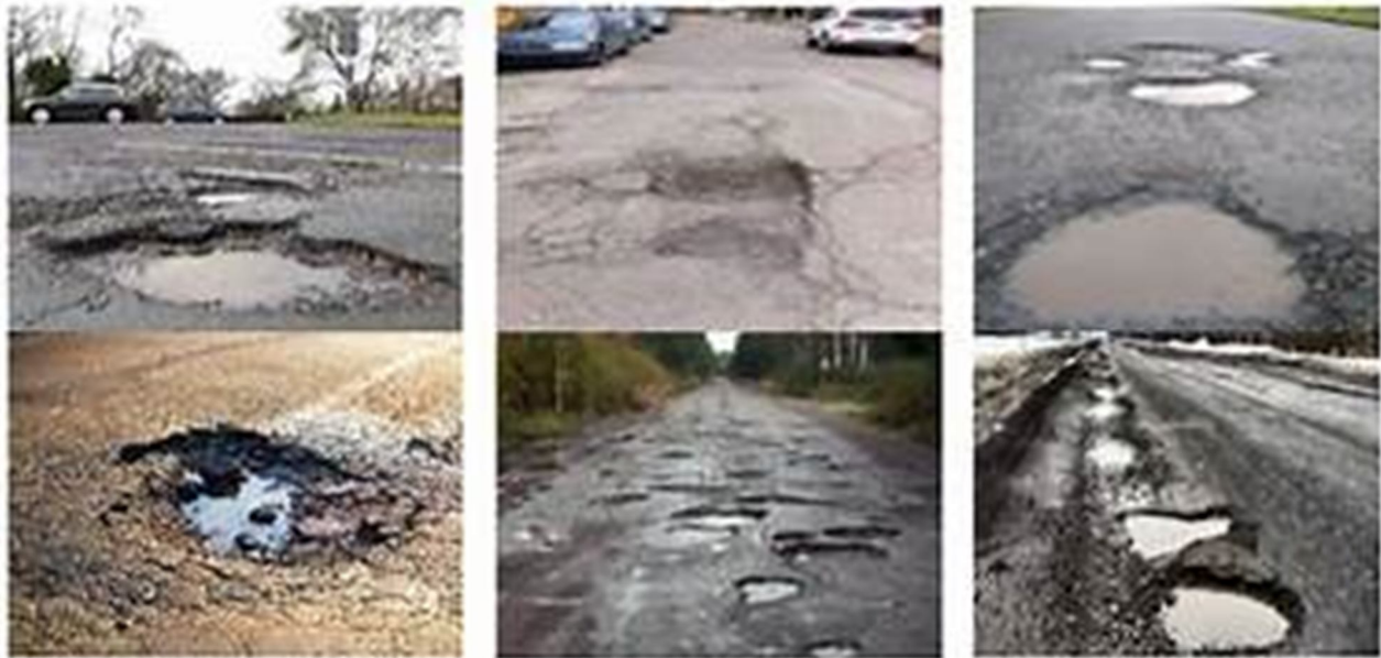
Figure 7 : Typical pothole images on road surfaces of the testing subset.
