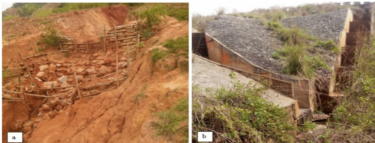
Fig.1.1: Different technical methods used mitigate soil erosion and slope failures in the biggest gully site in South eastern (Nigeria): (a) sand bags (b) runoff breakers (Igwe and Una 2019).
