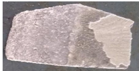
Figure 6: Sulphate Attack of Brick
