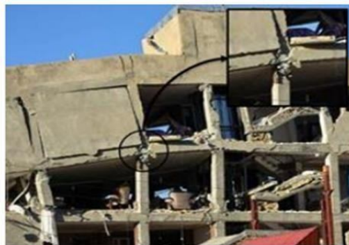
Fig. 1 Joint shear failure in the damaged buildings after the Kermanshah earthquake
