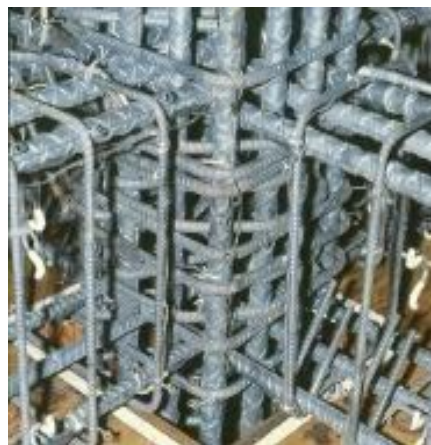
Fig. 3 Reinforcement steel congestion at the beam column joint
