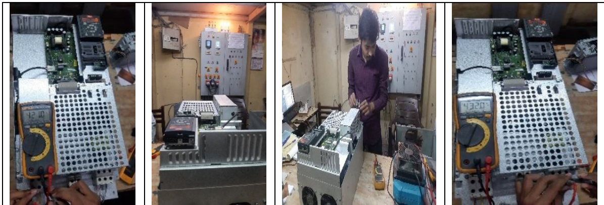
Fig.3 Hot test (power panel through) of VFD
