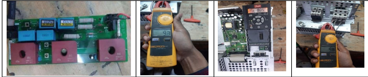
Fig.13 power panel through hot test of CT card
