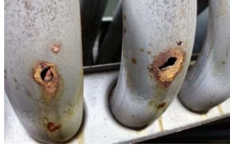
U Bend Erosion
