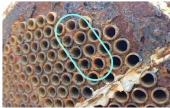
Inlet Tube End Erosion
