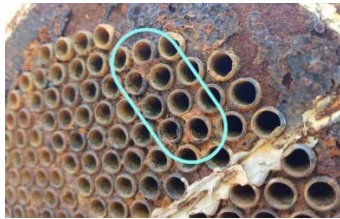
Inlet Tube End Erosion
