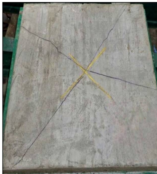
Fig. 4: Crack Pattern in slab
