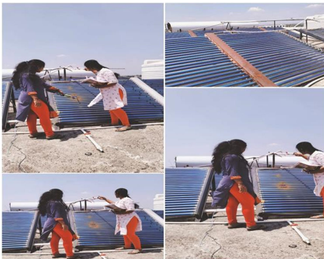
Fig6.1: Assessment of solar panel of hostel.
