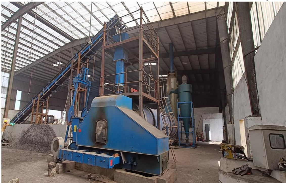
Figure-2 .Main View of Rotary Dryer
