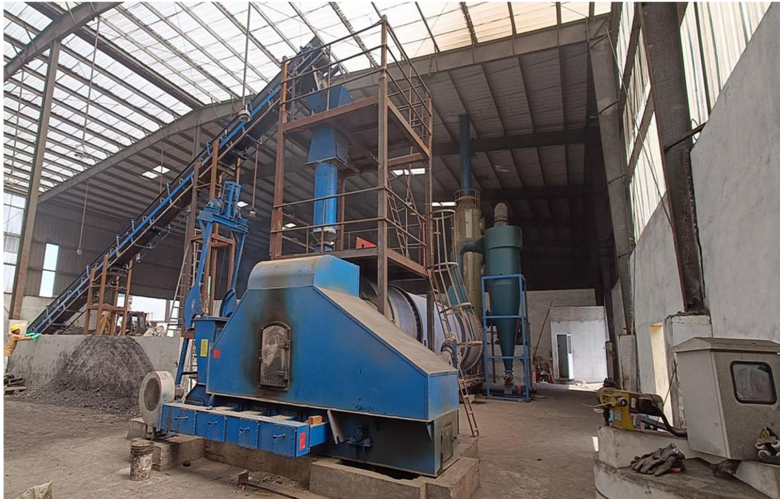
Figure-2 .Main View of Rotary Dryer
