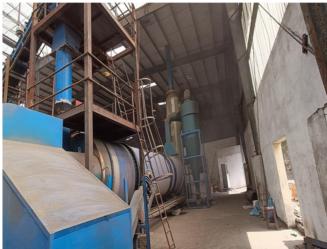
Figure-3. Side View of Rotary Dryer
