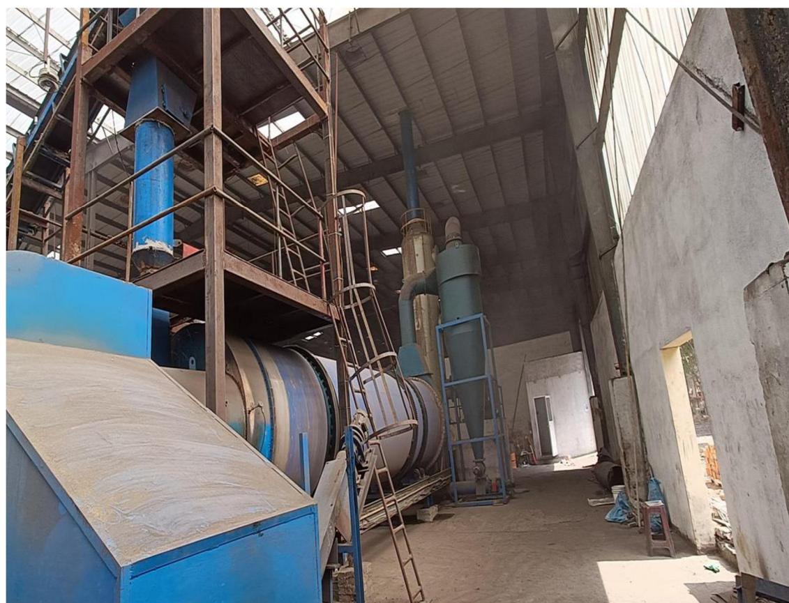
Figure-3. Side View of Rotary Dryer
