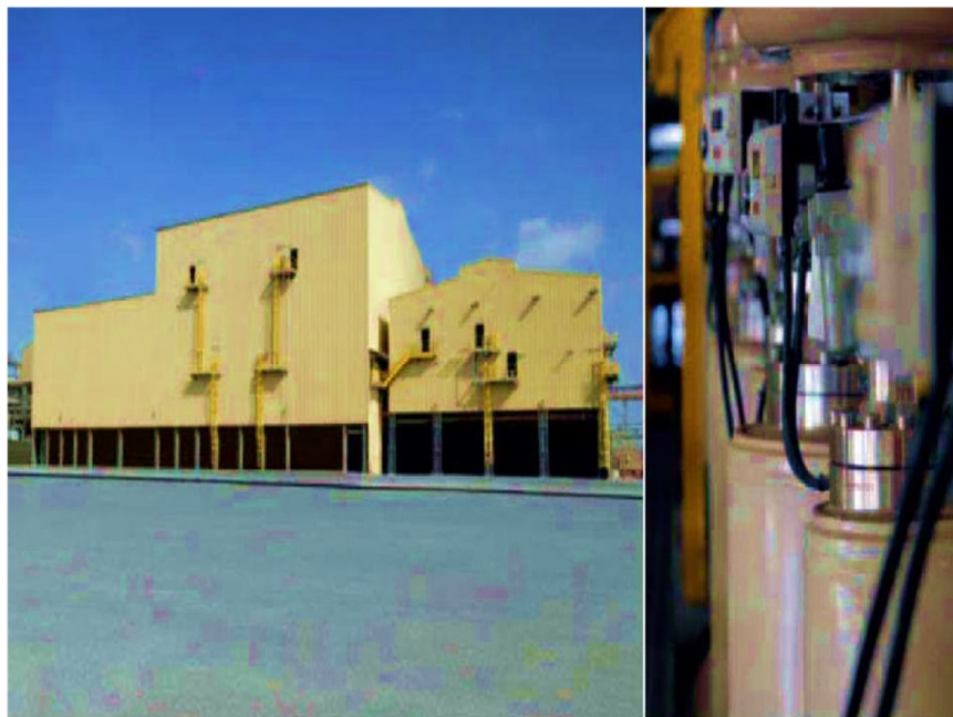
Fig 8: Conventional Helium Recovery – Helium Project of Rasgas
