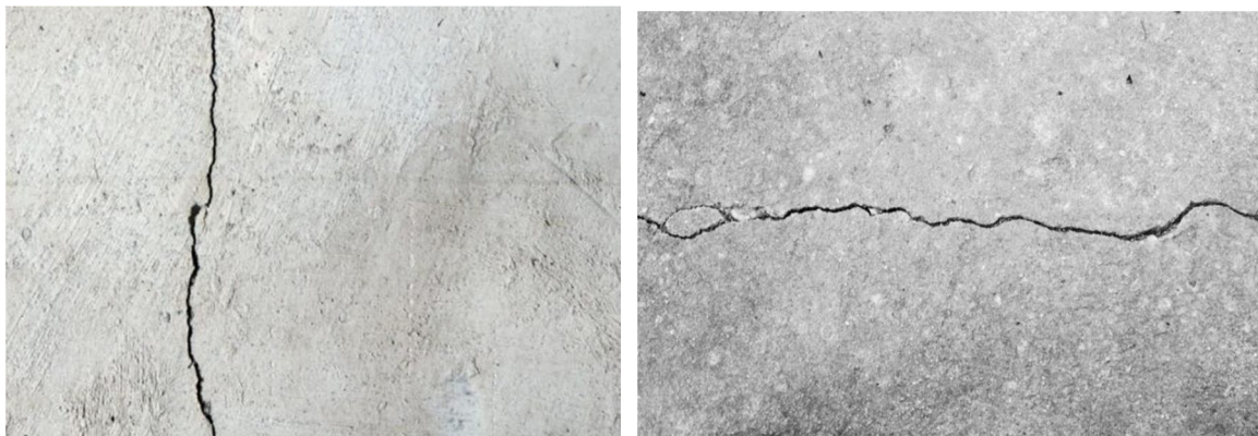
Figure 1. Sample image of crack.
