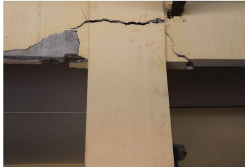
Fig. 3. Site Beam and Column Cracking
